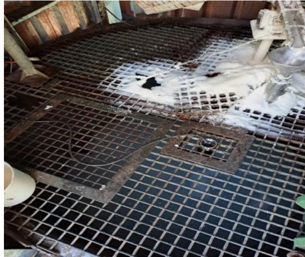
Figures 16. An uncovered mixing tank exposed to foreign matter ingress
