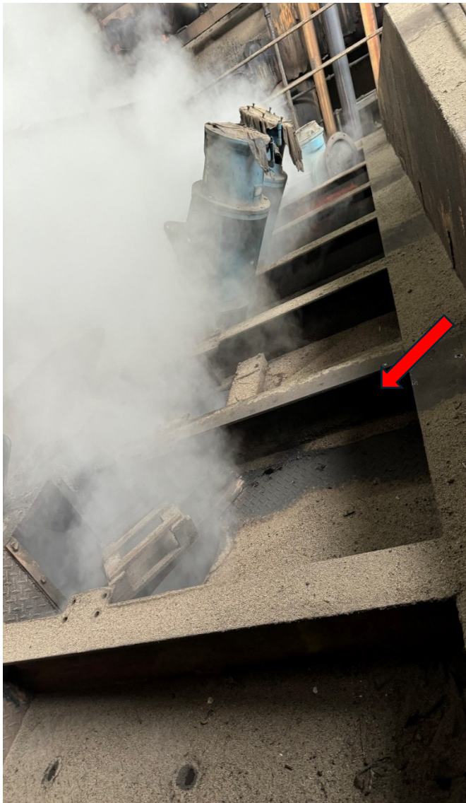
Figure 5. A representation of how steam leaks prevented maintenance from being done on the screws, while the diffuser is in operation
