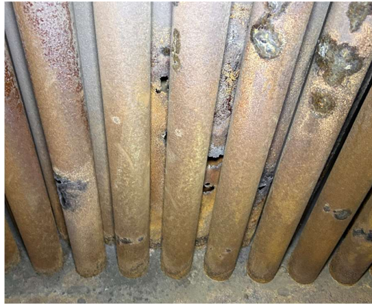
Figure 5. Corroded air heater tubes
