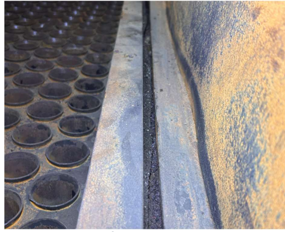
Figure 4. Defective air heater rope seal
