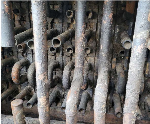
Figure 7. Economiser with six elements blanked off
