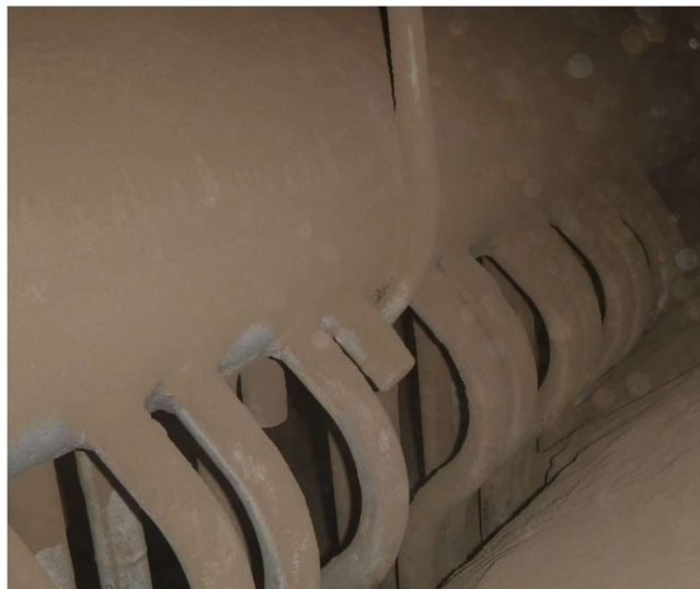
Figure 6. Missing superheater elements visible at the steam outlet header
