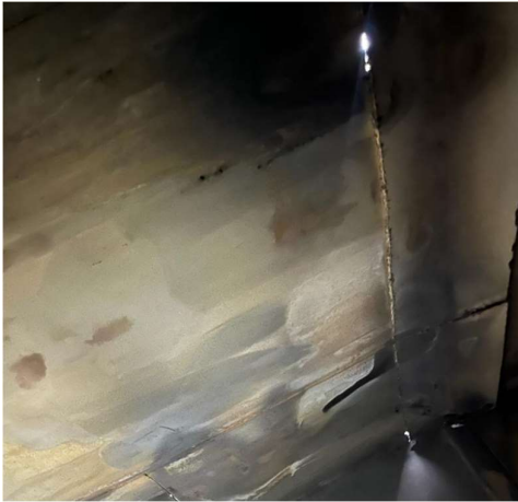
Figure 3. Failed air heater casing
