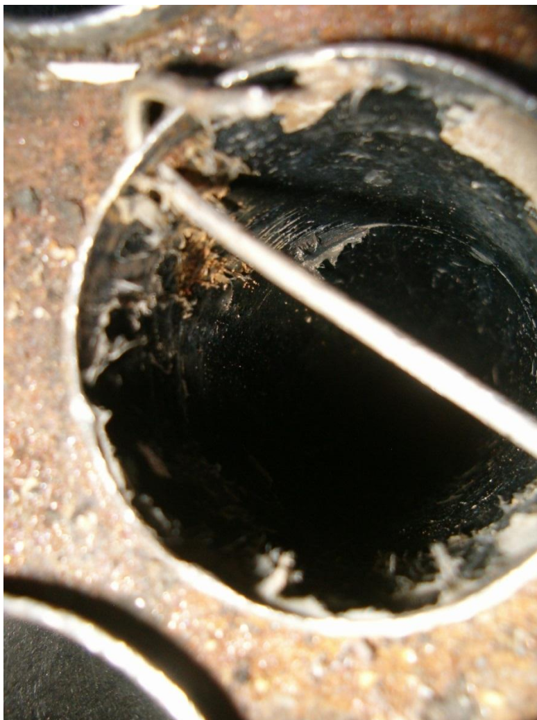
Figure 3. Tube appearance after a complete season without cleaning. The coating is peeling where scratched by the tube expander and at the tube extremes, but scale accumulation is negligible.
