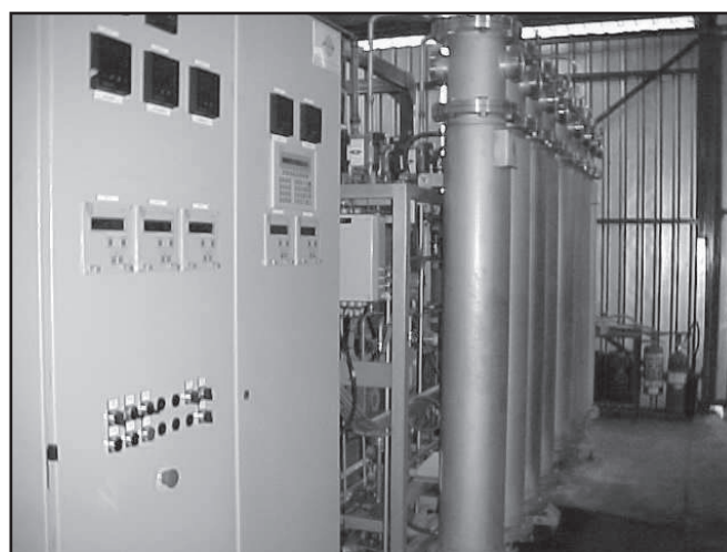
Figure 2. A view of the Chromatography Pilot Plant as installed.
