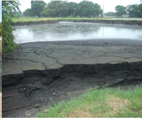
Figure 3. Dam 1 silt accumulation.
