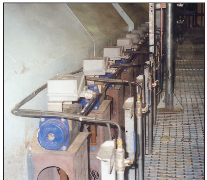
Figure 7. View of TES auto-controlled zoning damper operating gear.
