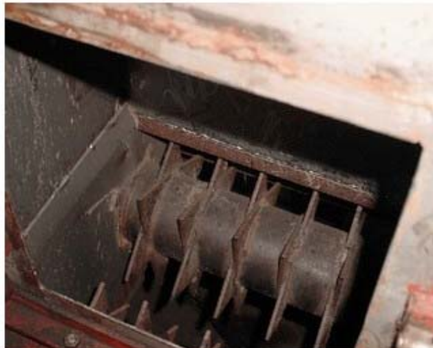
Figure 2. Bottom of NIR chute at Maidstone DAC station, looking through the trapdoor at discharge rolls.
