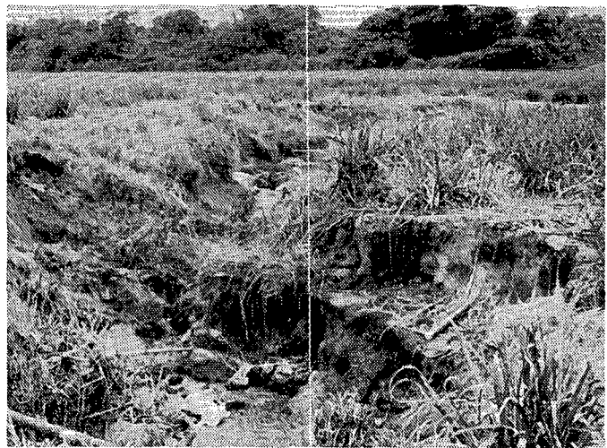
FIGURE 5 Streambank erosion showing banks collapsing due to undercutting action of the stream.
